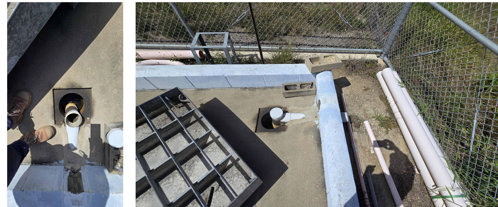
IMAGES OF EXISTING OIL SEPERATOR TO BE REPLACED WITH NEW
