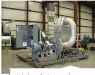
Maintaining exhaust systems on machines
