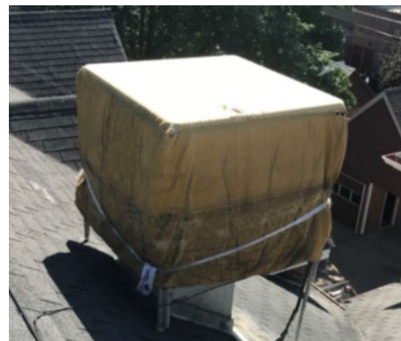
Example Evaporative Cooler with Cover
