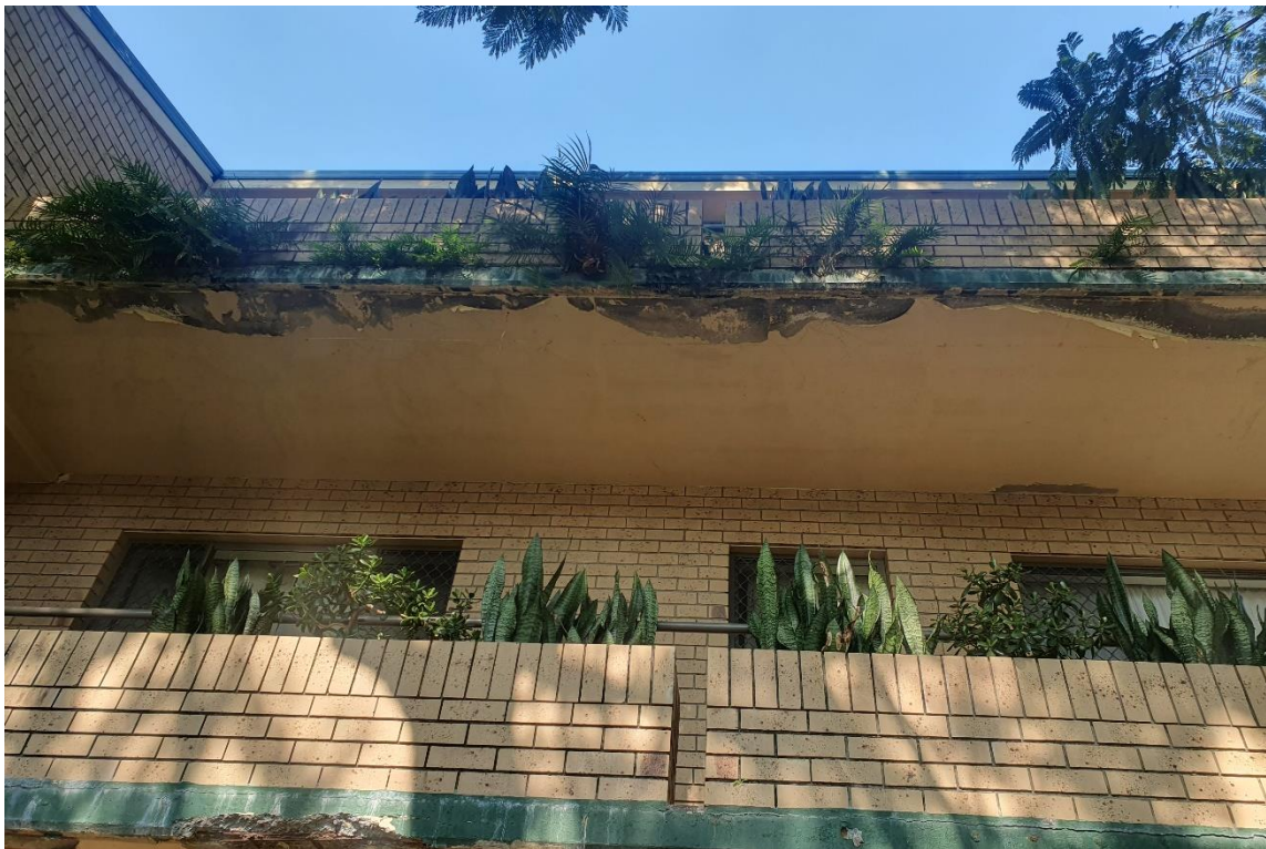
PHOTOGRAPH 6.: Minor areas of reinforcement exposure/ concrete cancer. Paint has significant spalling/ peeling
