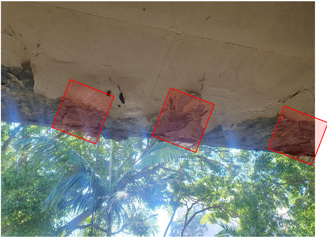
PHOTOGRAPH 17.: Moderate cracking to concrete slab, evidence of early spalling/ blow-out from concrete cancer
