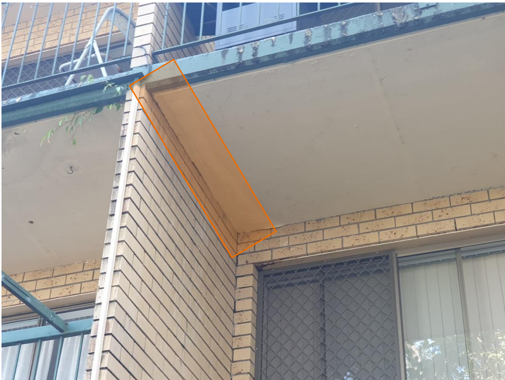
PHOTOGRAPH 34.: Concrete slab expansion alongside brick support
