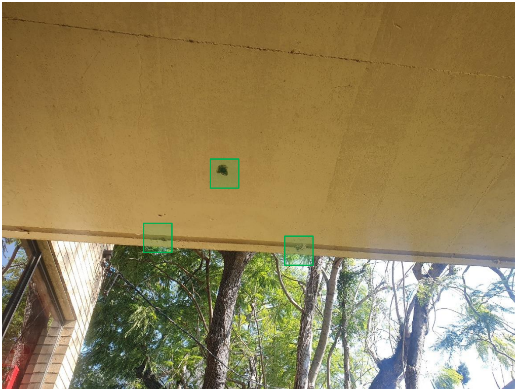
PHOTOGRAPH 27.: Minor defects to underside bridge, minor areas of spalling/ paint deterioration
