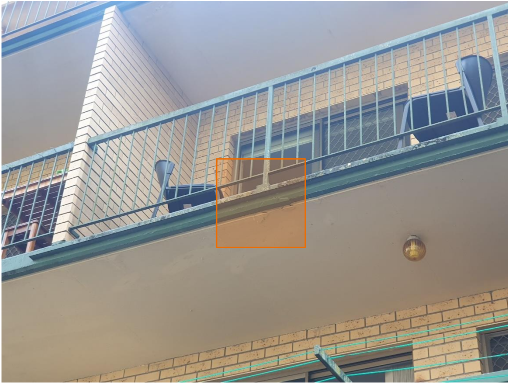
PHOTOGRAPH 33.: Minor spalling/ blow out of concrete slab
