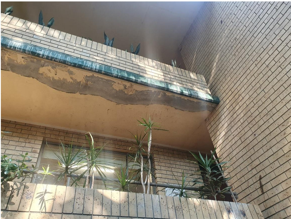
PHOTOGRAPH 14.: no indication of slab spalling/ cracks. Paint work has peeled away in large sections
