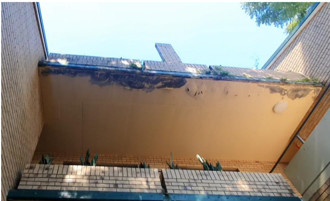
PHOTOGRAPH 10.: Some spalling of concrete, areas of paint fully deteriorated.
