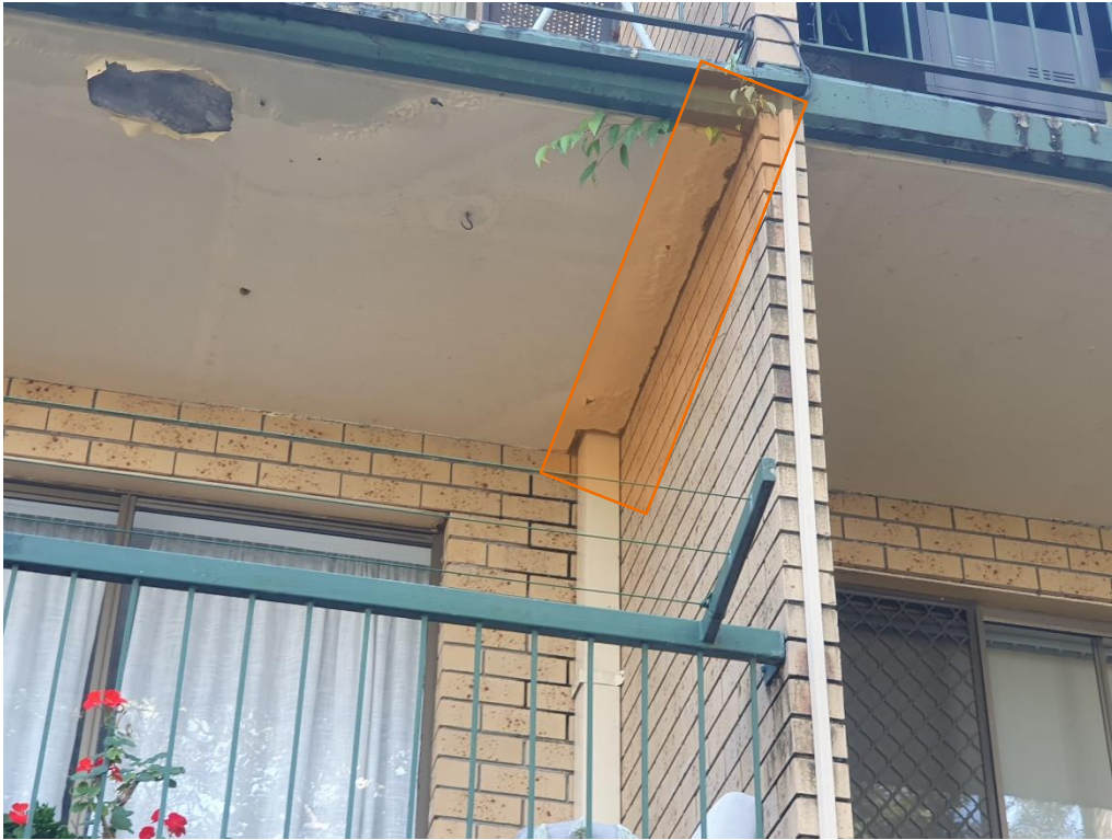
PHOTOGRAPH 35.: Concrete slab expansion alongside brick support
