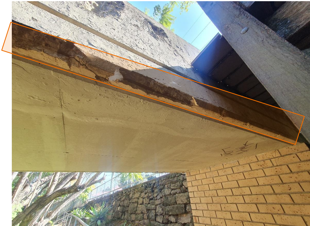
PHOTOGRAPH 23.: Underside bridge, moderate concrete cancer. Concrete spalling/ deterioration along underside edge
