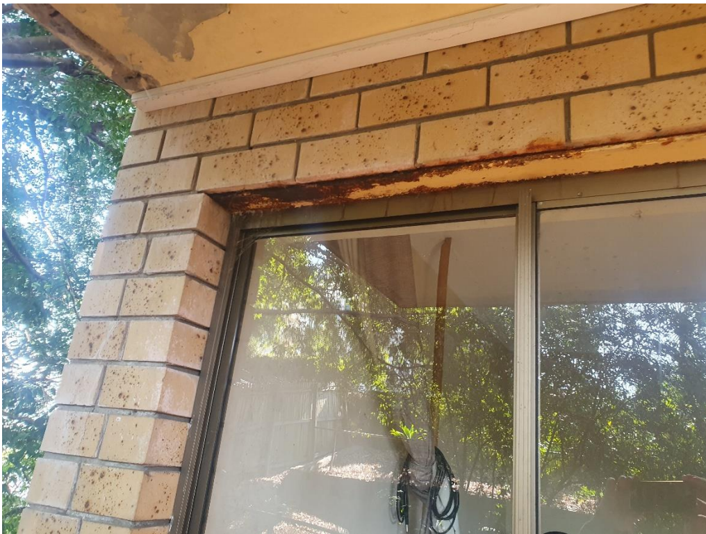
PHOTOGRAPH 16.: Moderate corrosion to steel window lintel
