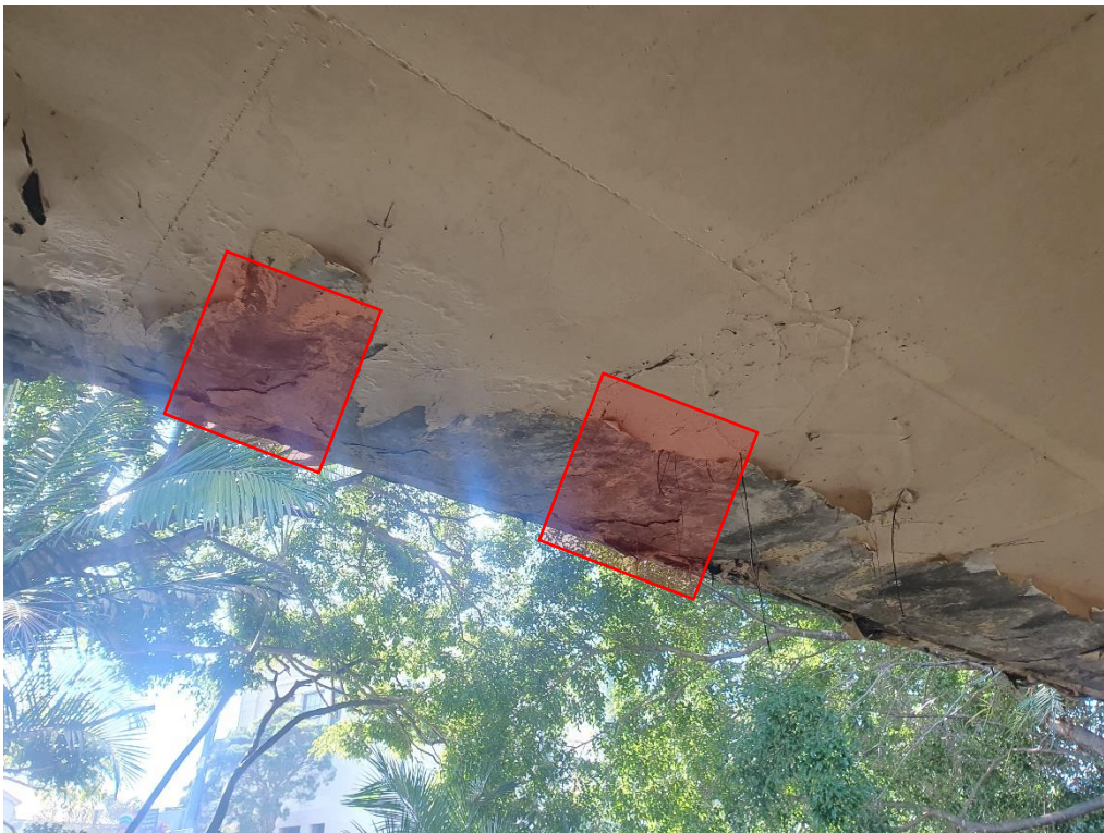
PHOTOGRAPH 18.: Moderate cracking to concrete slab, evidence of early spalling/ blow-out from concrete cancer
