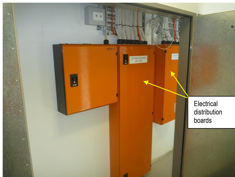
Figure 18.1 Typical EDB cupboard – photo 1
