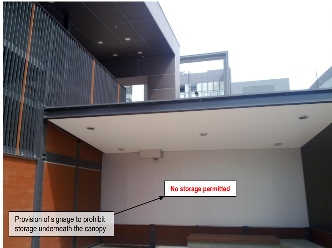
Figure 18.9 Non-sprinkler protected canopy in courtyard (proposed wording for signage)
