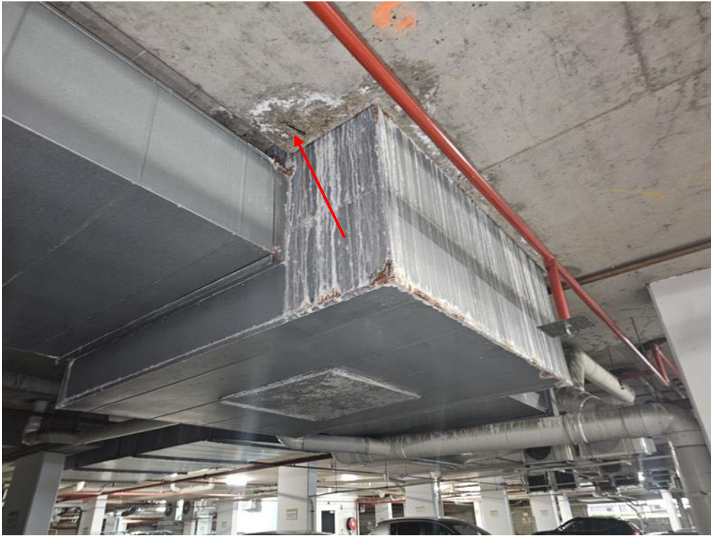
PHOTOGRAPH 5.: Defect Class B: Reinforcement exposed due to concrete spalling
