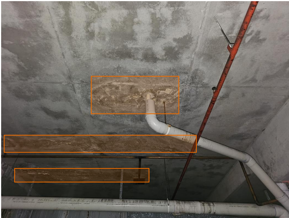
PHOTOGRAPH 7.: Defect Class B: Large area of straining, early stage of steel corrosion
