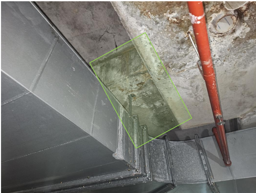
PHOTOGRAPH 14.: Defect Class A: Visible staining of concrete, some efflorescence visible, no visible cracking or spalling of concrete
