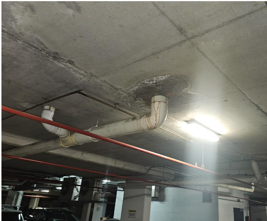
PHOTOGRAPH 15.: Defect Class A: Visible staining of concrete, some efflorescence visible around pipe penetration
