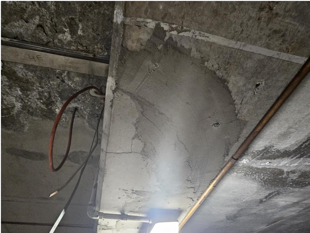
PHOTOGRAPH 20.: Defect Class C: Previous surface repairs evident
