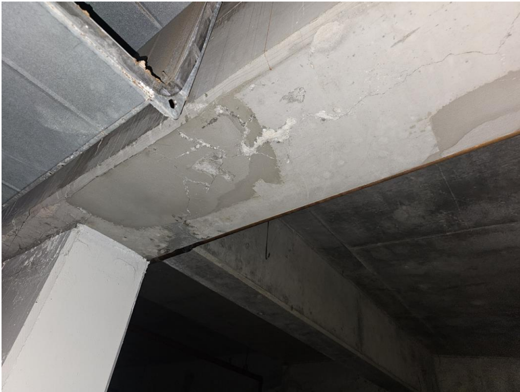
PHOTOGRAPH 18.: Defect Class C: Previous surface repairs evident
