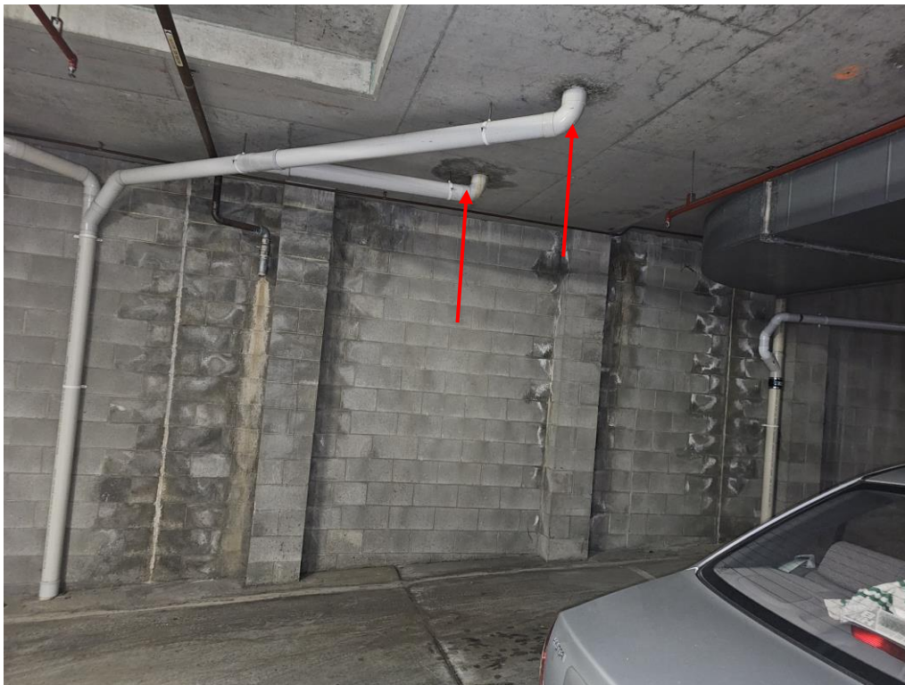
PHOTOGRAPH 4.: Defect Class A: Staining to concrete around pipe penetrations. Wall also indicates water penetration with notable efflorescence to the block wall
