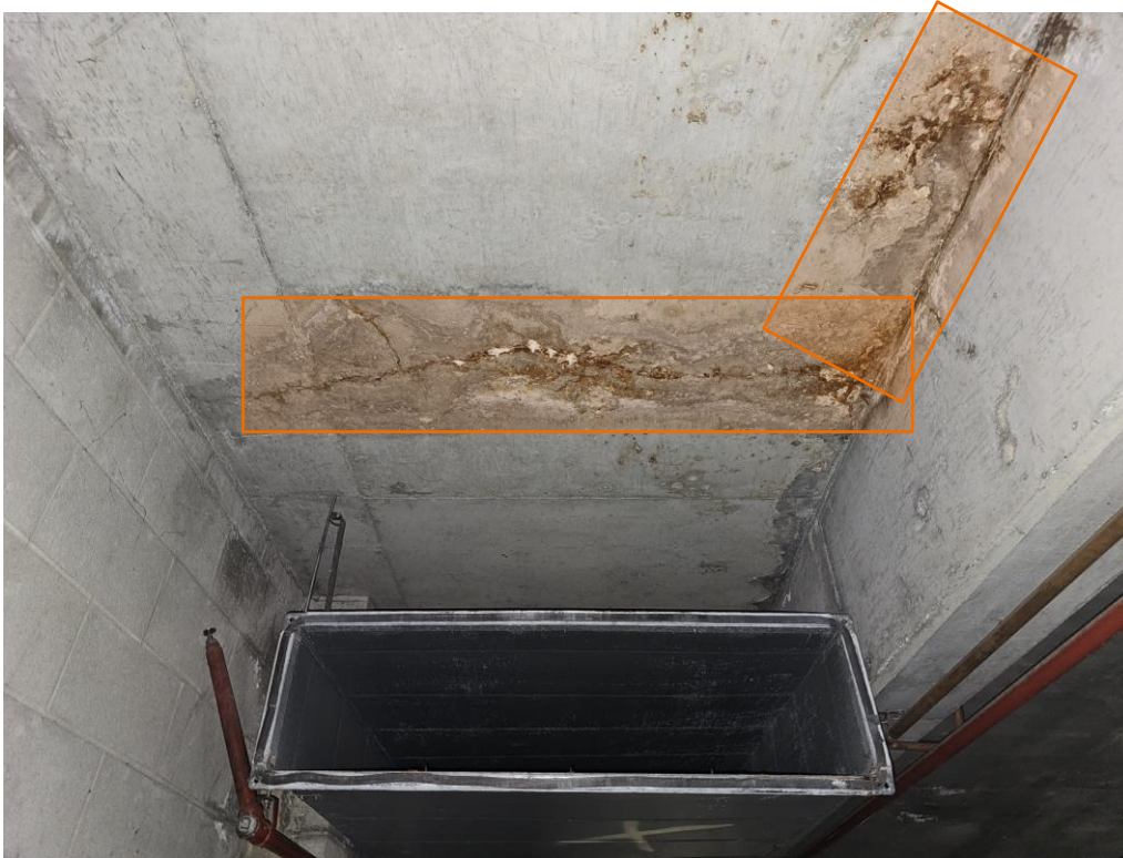
PHOTOGRAPH 11.: Defect Class B: Large area of straining, cracking to concrete surface
