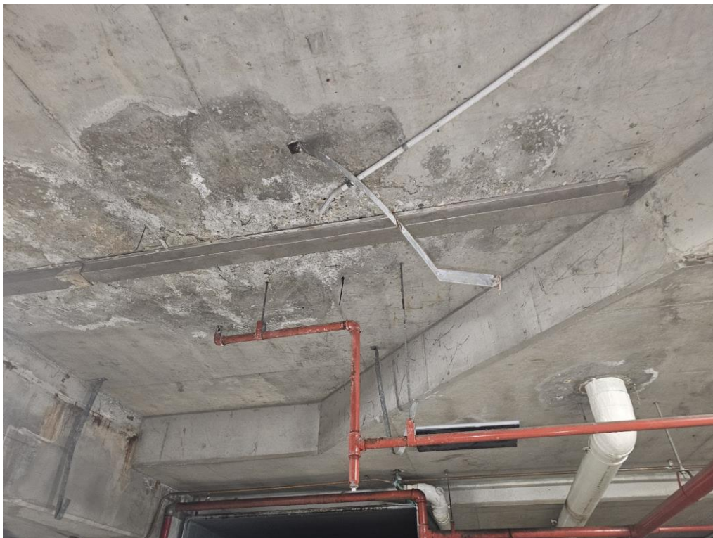
PHOTOGRAPH 16.: Defect Class B: Visible staining of concrete, some efflorescence visible, some spalling of concrete along drip tray
