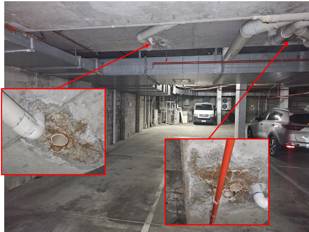
PHOTOGRAPH 13.: Defect Class A: Visible staining of concrete, some efflorescence visible
