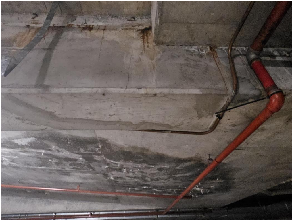
PHOTOGRAPH 19.: Defect Class C: Moderate cracking & spalling to concrete beam, beam supports pool above. Cracking depth up to 200mm into depth of beam
