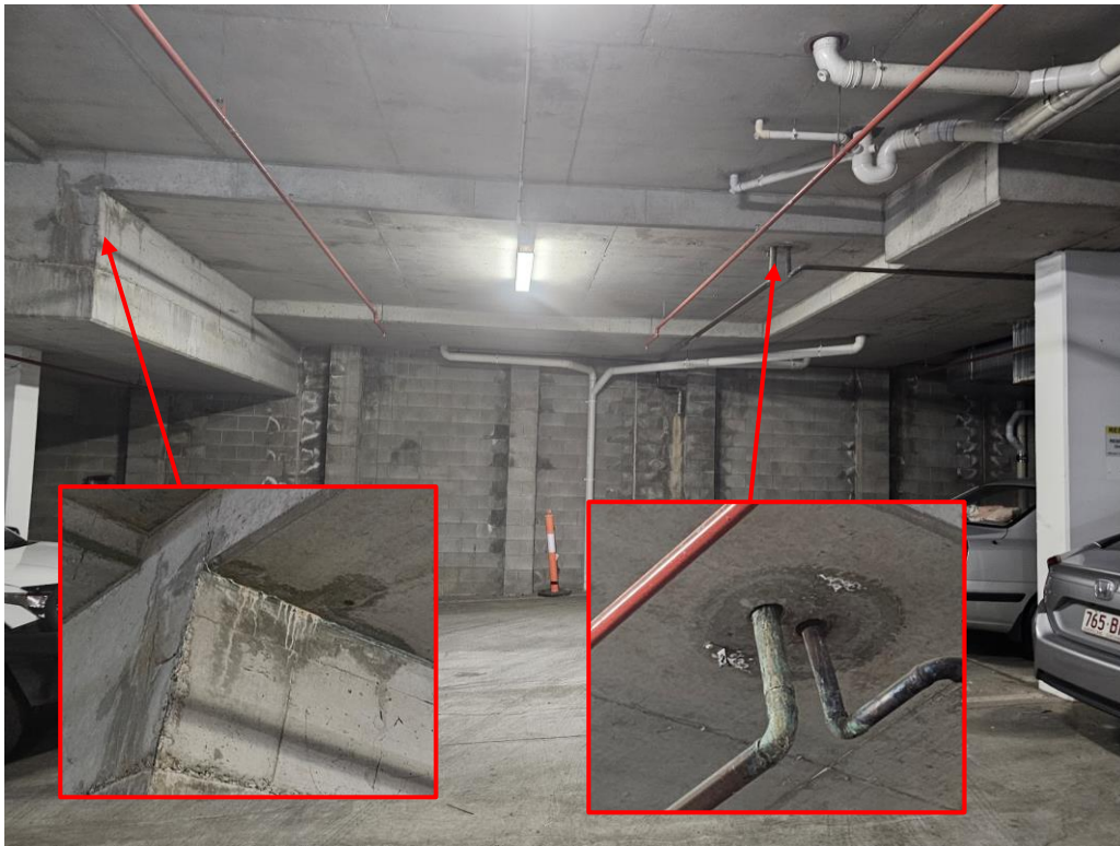
PHOTOGRAPH 1.: Defect Class A: Visible staining of concrete, some efflorescence visible
