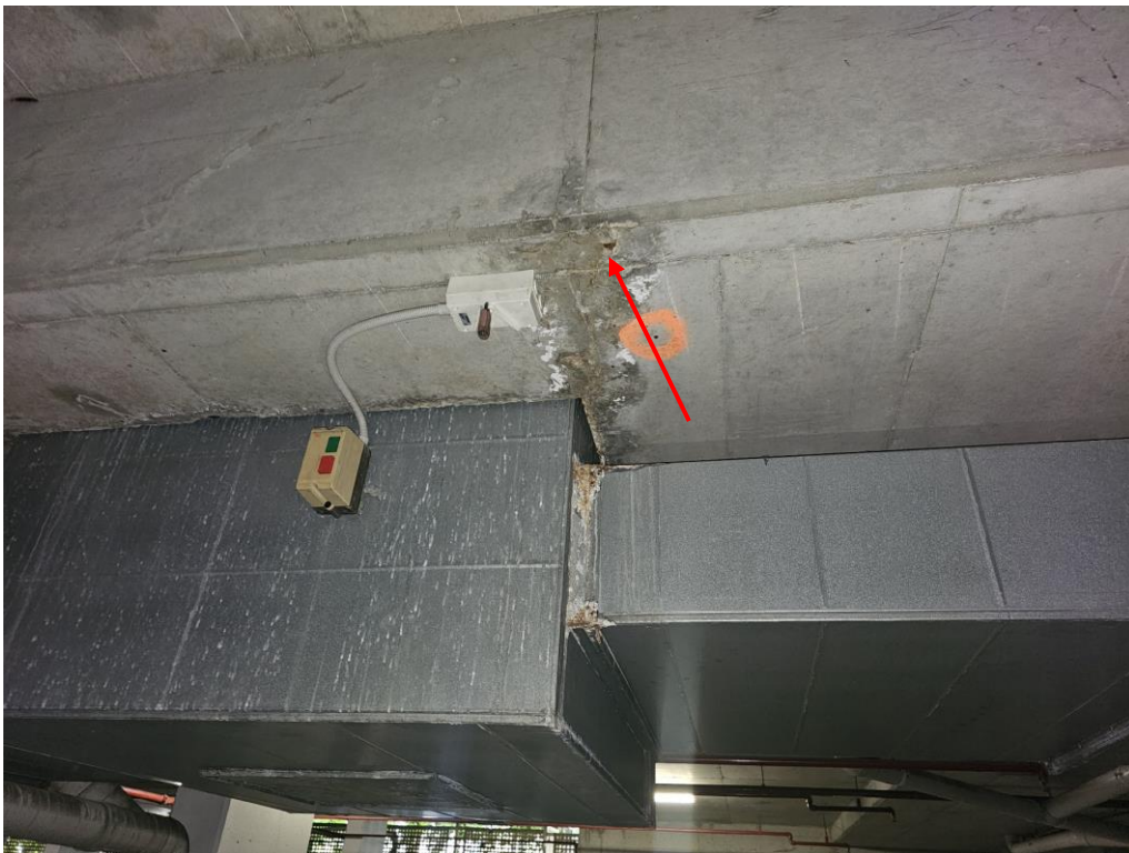
PHOTOGRAPH 6.: Defect Class B: Reinforcement exposed due to concrete spalling
