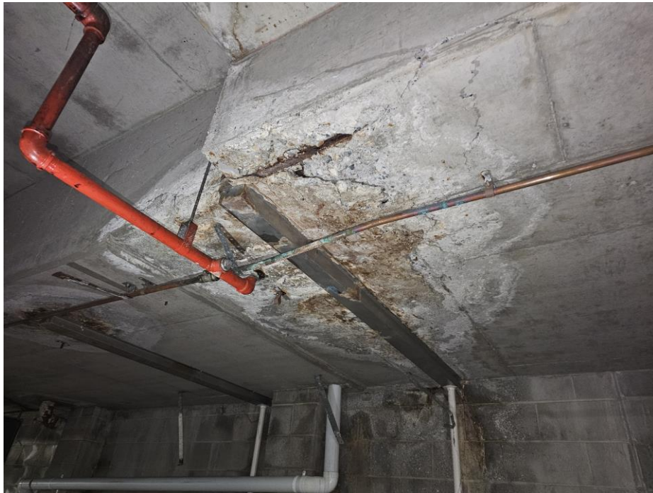
PHOTOGRAPH 10.: Defect Class C: large cracks across concrete face, large are of spalling with multiple chunks of concrete falling away to expose aggregate
