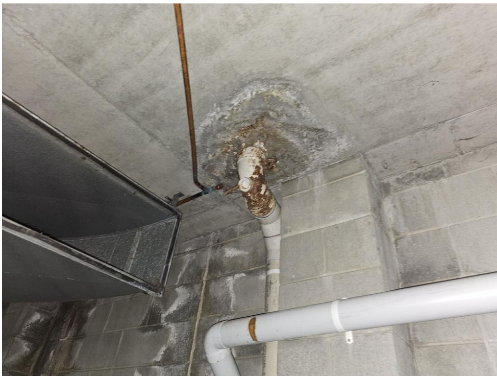
PHOTOGRAPH 8.: Defect Class A: Staining & material deposits to concrete around pipe penetration
