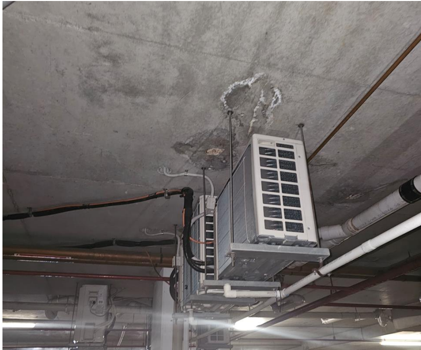
PHOTOGRAPH 3.: Defect Class A: Visible staining of concrete, located around air con
