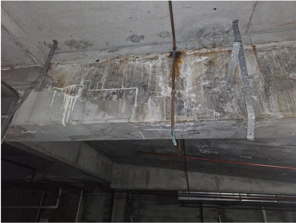
PHOTOGRAPH 17.: Defect Class C: Moderate cracking & spalling to concrete beam, beam supports pool above. Cracking depth up to 200mm into depth of beam
