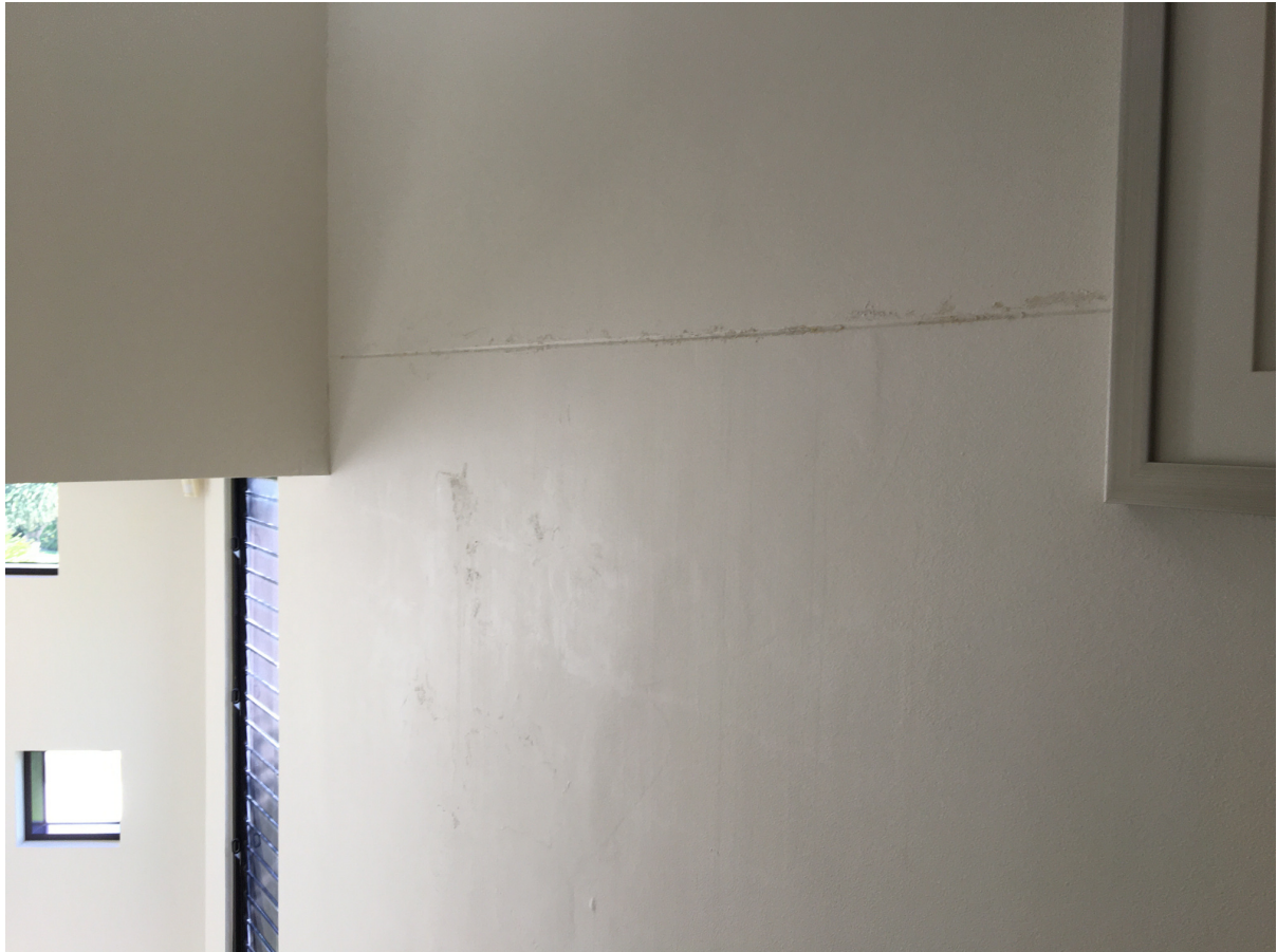
Internal water damage
