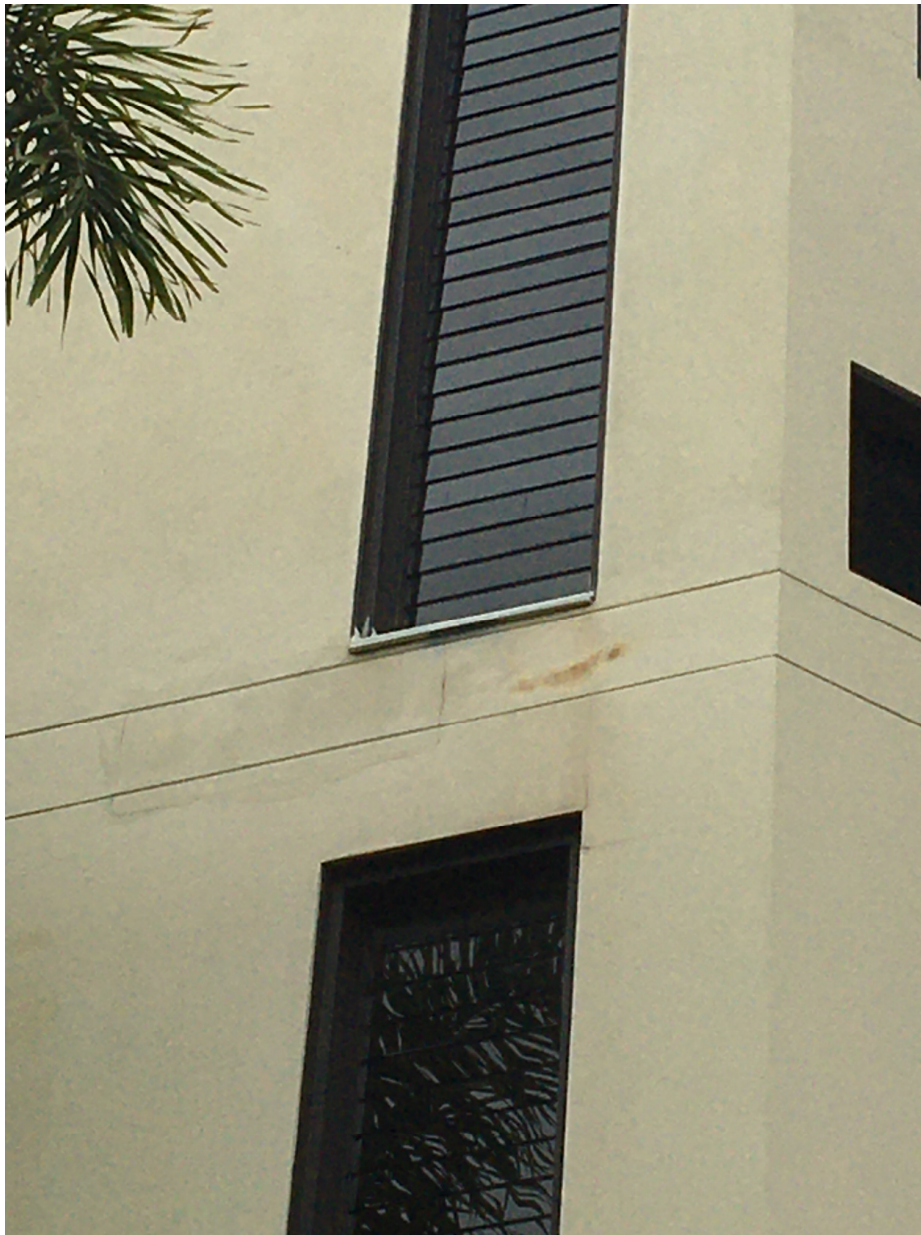
Existing external damage
