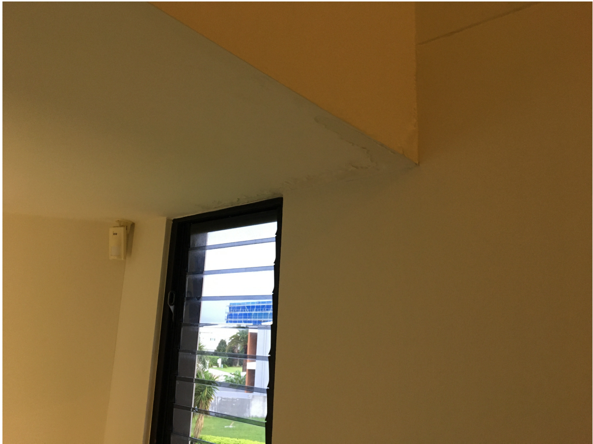
Internal water damage
