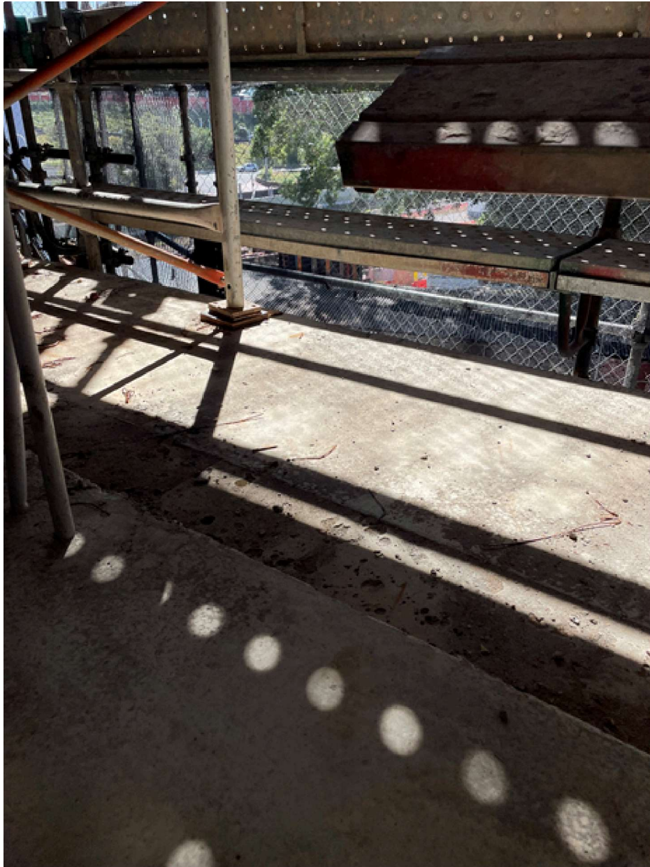
View from a suspended slab, inside the building looking out; the rebate (stepdown) visible in the bottom of the photo is too small
