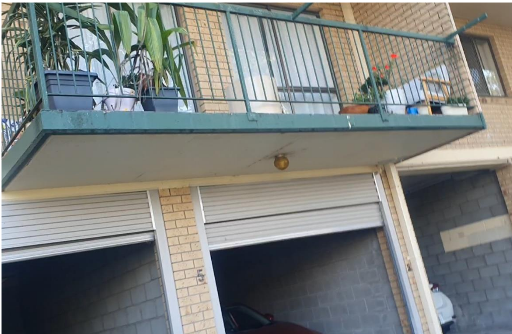
PHOTOGRAPH 30.: No evidence of concrete cancer, minor indications of deterioration. Minor defects to paint coating
