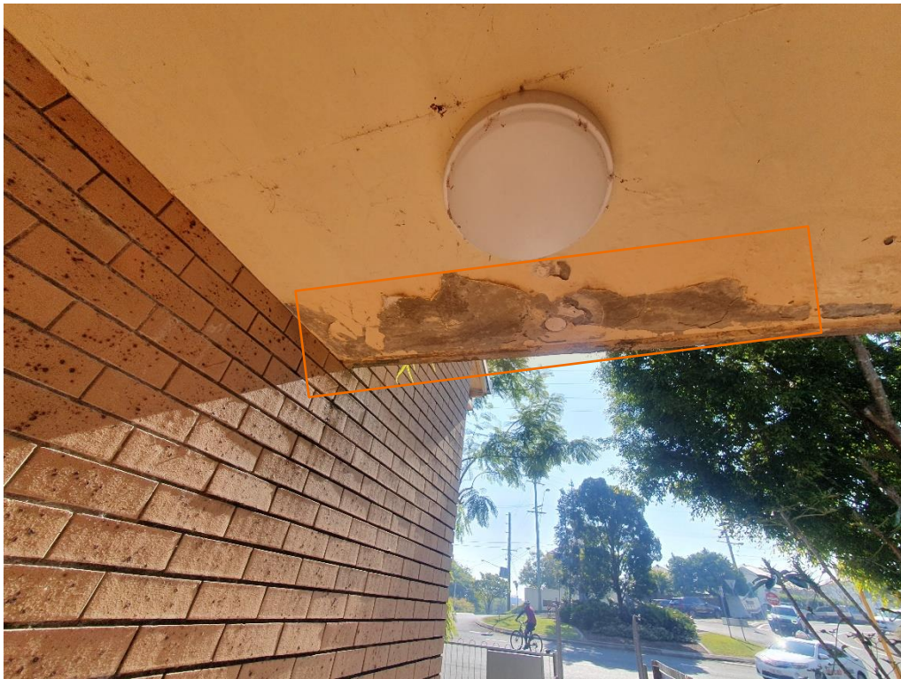
PHOTOGRAPH 11.: cracking to concrete slab, spalling to some areas.
