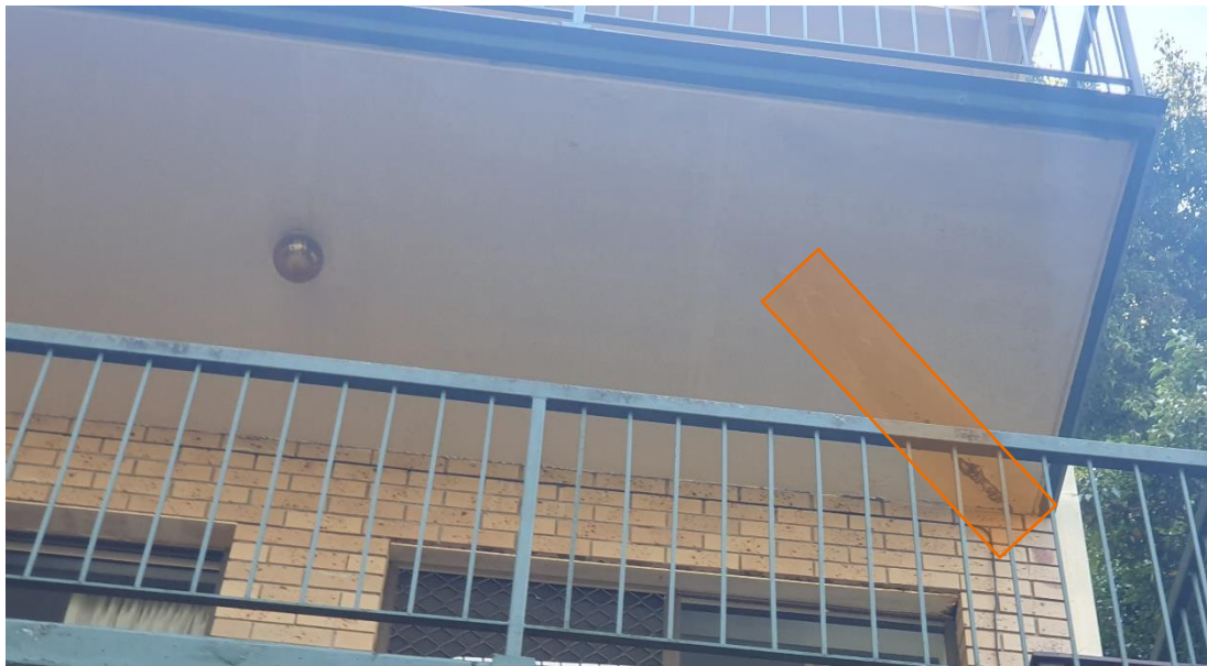
PHOTOGRAPH 38.: Long dark stain/ crack indicates early reinforcement corrosion
