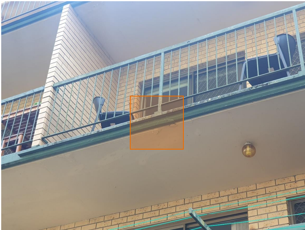
PHOTOGRAPH 33.: Minor spalling/ blow out of concrete slab
