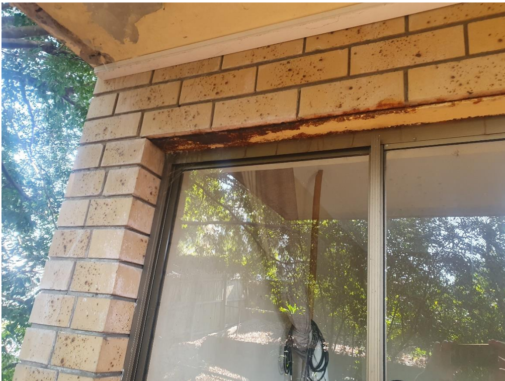
PHOTOGRAPH 16.: Moderate corrosion to steel window lintel
