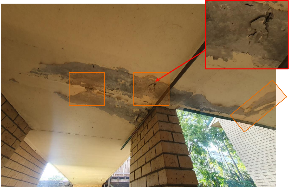
PHOTOGRAPH 9.: Below walkway above concrete spalling/ falling away in small sections
