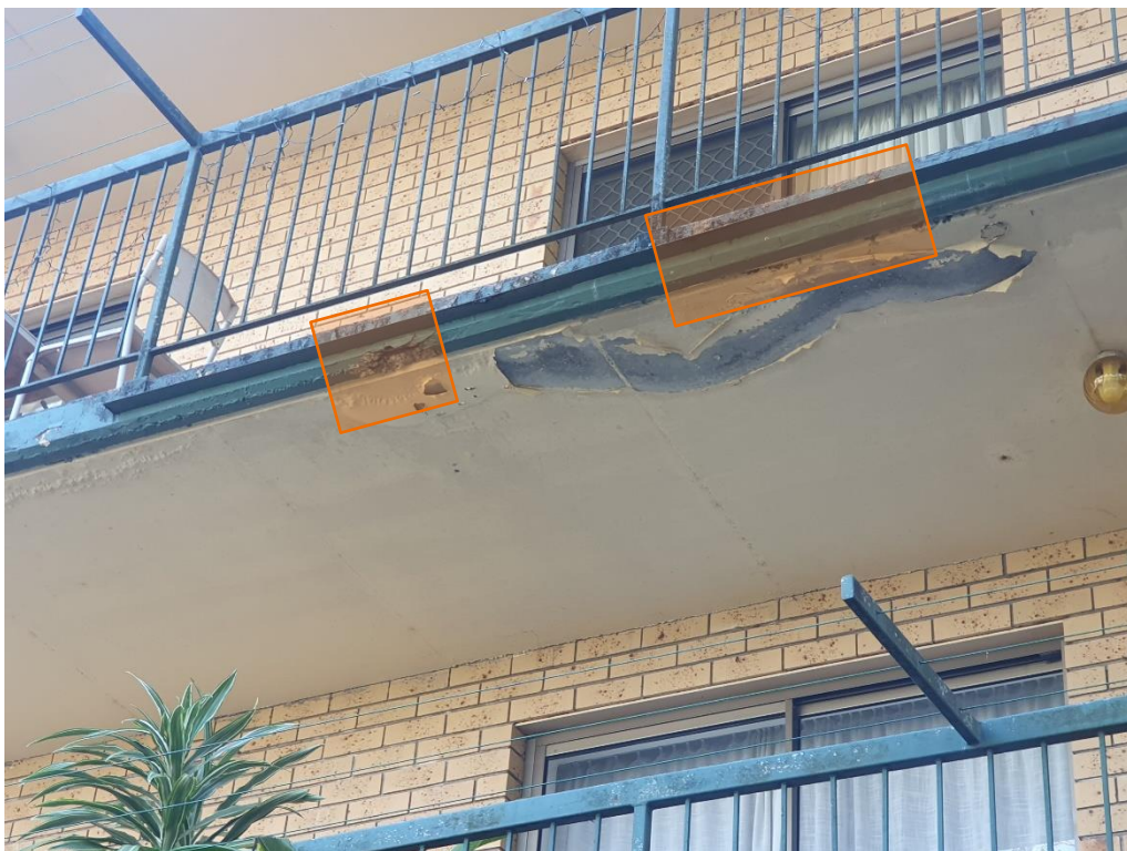
PHOTOGRAPH 36.: Sections/ chunks of concrete slab have fallen away, sections of reinforcement corroded/ exposed
