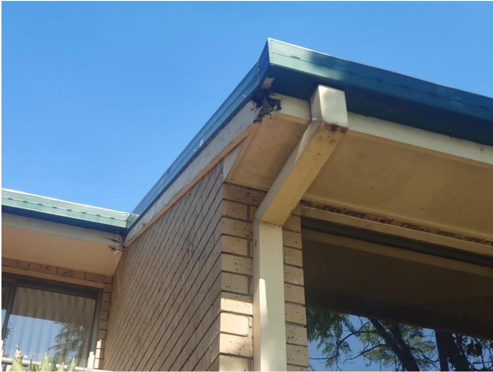
PHOTOGRAPH 21.: Severe timber rot to timber skirting along roof eave
