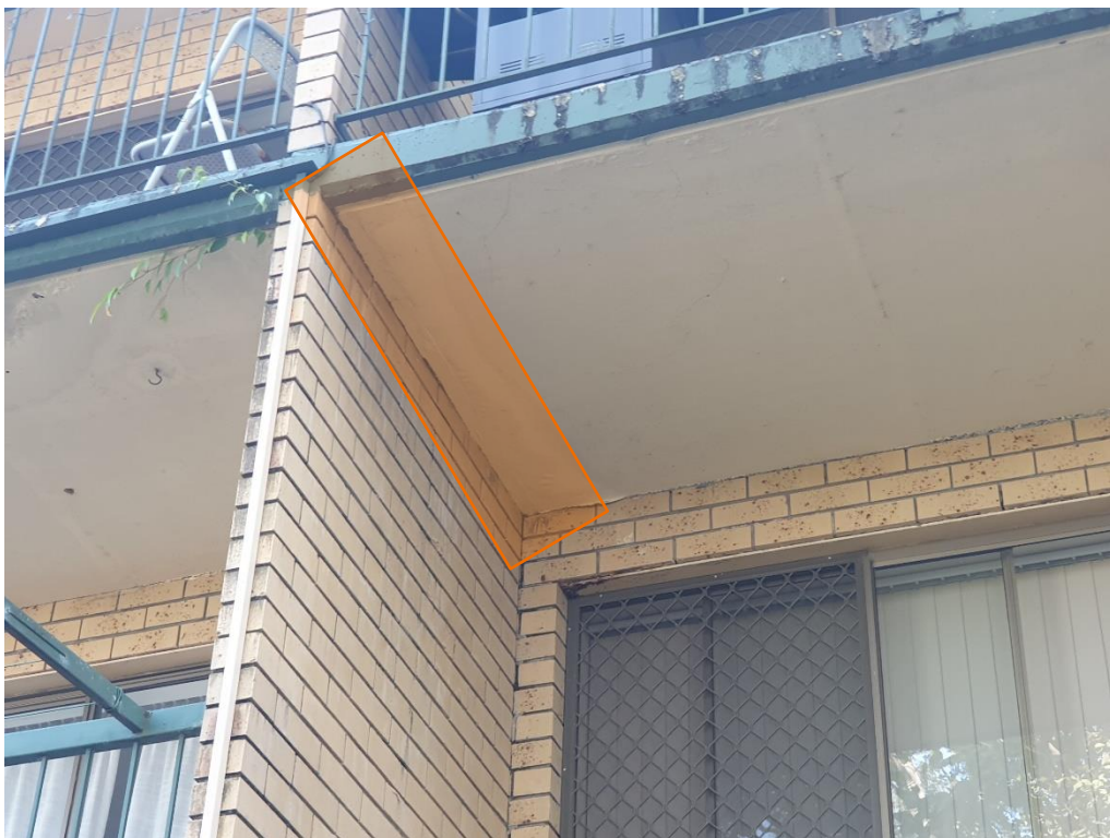
PHOTOGRAPH 34.: Concrete slab expansion alongside brick support
