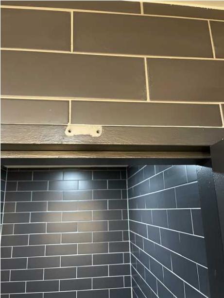
Photo 2 - Details Need door closer on middle door
