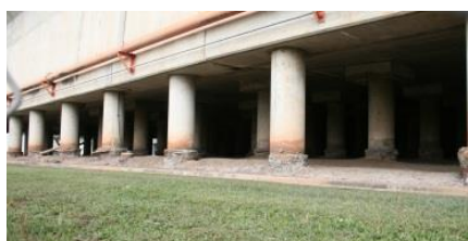
Figure 15: Acid damage to concrete structures
