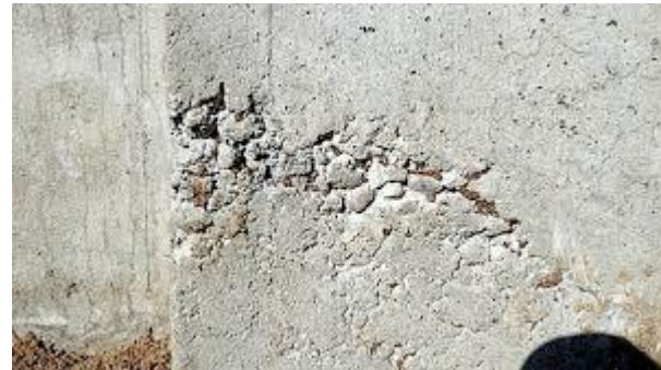
Example of honeycomb in concrete
