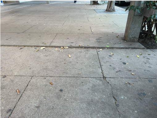
TYPICAL LIFTED / LIPPED CONCRETE FOOTPATH FOR CUTTING / GRINDING.
