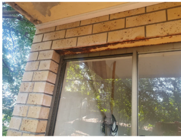
PHOTOGRAPH 16: Moderate corrosion to steel window lintel
