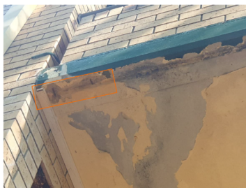
PHOTOGRAPH 15: Small area of exposed reinforcement, some minor slab spalling/ deterioration
