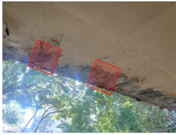
PHOTOGRAPH 18: Moderate cracking to concrete slab, evidence of early spalling/ blow-out from concrete cancer
