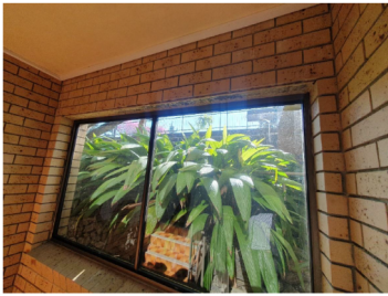
PHOTOGRAPH 20: Minor corrosion to steel window lintel
