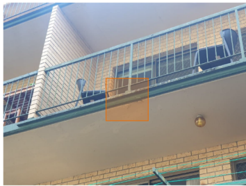
PHOTOGRAPH 33: Minor spalling/ blow out of concrete slab
