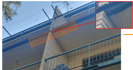
PHOTOGRAPH 39: Sections/ chunks of concrete slab have fallen away, sections of reinforcement corroded/ exposed
