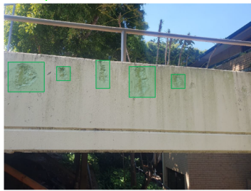
PHOTOGRAPH 25: Spalling of concrete wall over bridge, evident of concrete blow out due to concrete cancer
