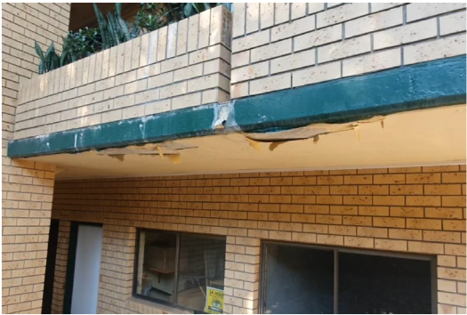
PHOTOGRAPH 7.: No evidence of concrete cancer, some efflorescence to concrete, paint is spalling/peeling
