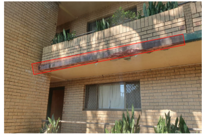
PHOTOGRAPH 4: Concrete cancer to balcony slab, extends back approx.400mm
