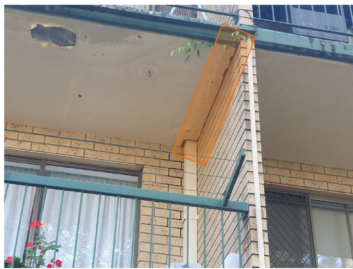
PHOTOGRAPH 35: Concrete slab expansion alongside brick support
