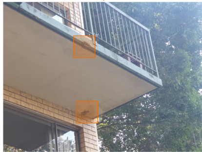
PHOTOGRAPH 31: Minor spalling/ blow out of concrete slab. Small area of reinforcement visible
