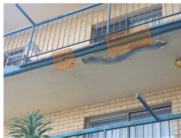
PHOTOGRAPH 36: Sections/ chunks of concrete slab have fallen away, sections of reinforcement corroded/ exposed
