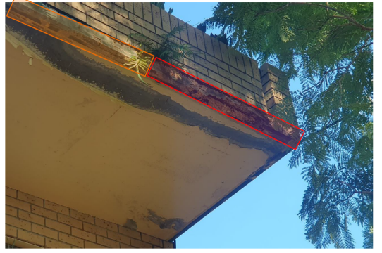
PHOTOGRAPH 5: Moderate concrete cancer 2.0m from corner along balcony.
