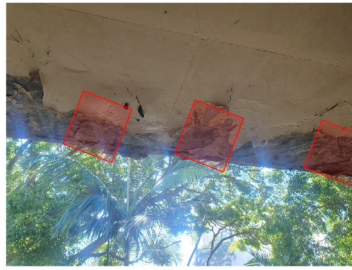
PHOTOGRAPH 17: Moderate cracking to concrete slab, evidence of early spalling/ blow-out from concrete cancer
