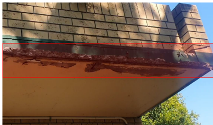
PHOTOGRAPH 3: Concrete cancer to balcony slab, extends back approx.400mm. Cancer along length of balcony at various points. Garden bed slab above slab
