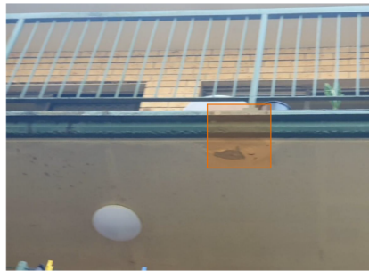
PHOTOGRAPH 32: Minor spalling/ blow out of concrete slab
