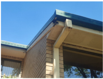
PHOTOGRAPH 21: Severe timber rot to timber skirting along roof eave
