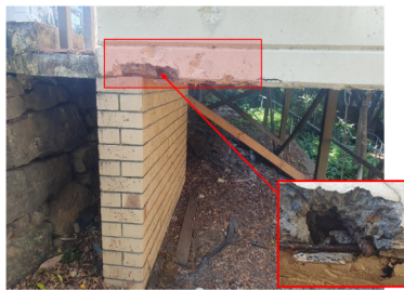
PHOTOGRAPH 24: Large void near bridge support wall, severe corrosion to reinforcement. Large chunks of slab are missing/ have fallen away
