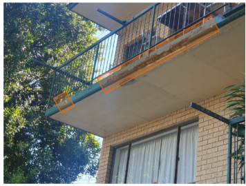
PHOTOGRAPH 37: Sections/ chunks of concrete slab have fallen away, sections of reinforcement corroded/ exposed
