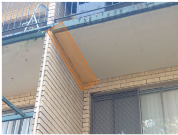
PHOTOGRAPH 34: Concrete slab expansion alongside brick support
