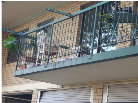
PHOTOGRAPH 29.: No evidence of concrete cancer, minor indications of deterioration. Minor defects to paint coating
