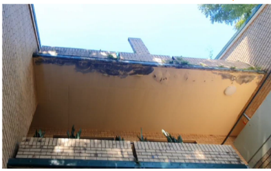
PHOTOGRAPH 10: Some spalling of concrete, areas of paint fully deteriorated.
