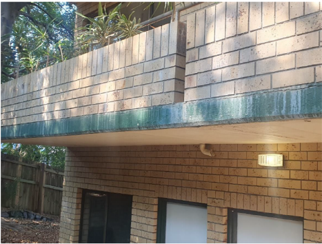
PHOTOGRAPH 13.: Slab in generally good condition, with some efflorescence, minor paint defects
