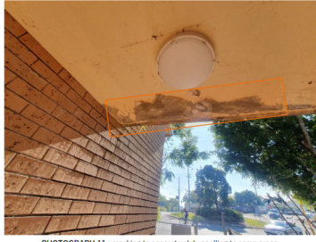
PHOTOGRAPH 11: cracking to concrete slab, spalling to some areas.
