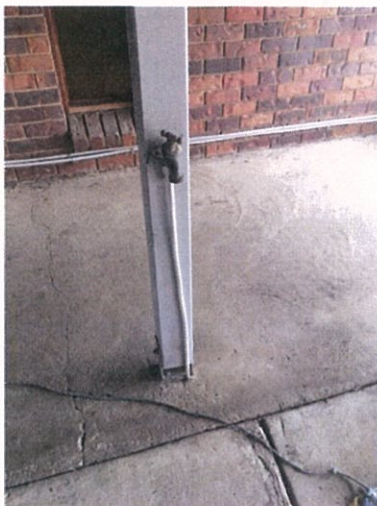
Delap cracks to concrete
