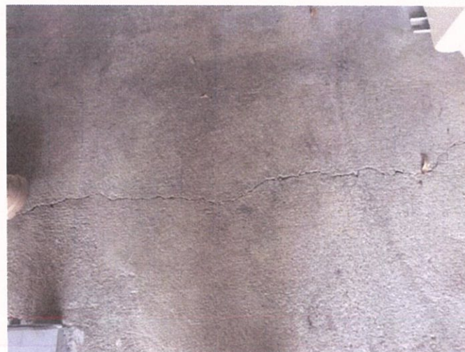
Delap cracks to concrete
