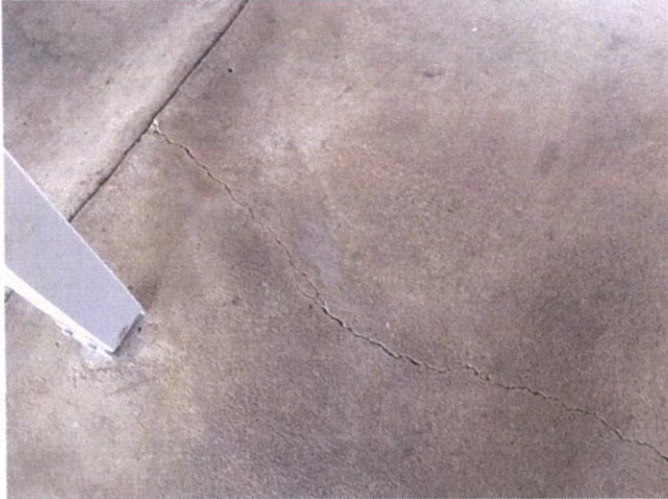
Delap cracks to concrete
