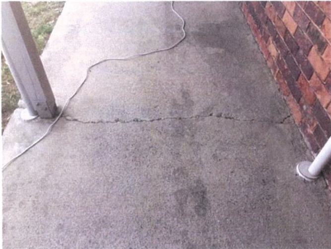
Delap cracks to concrete
