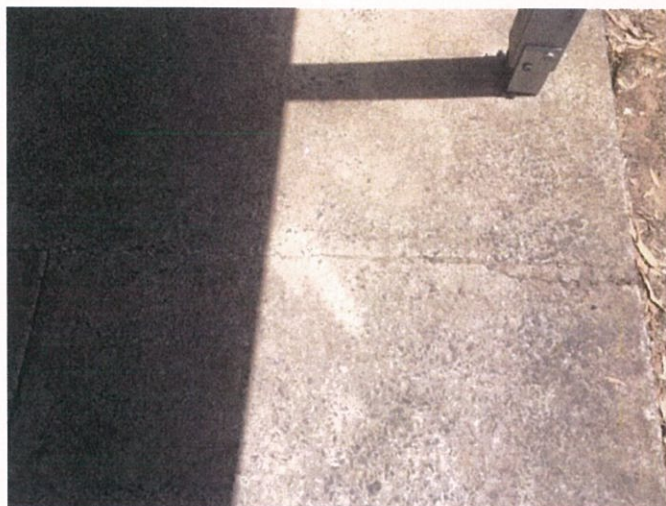
Delap cracks to concrete
