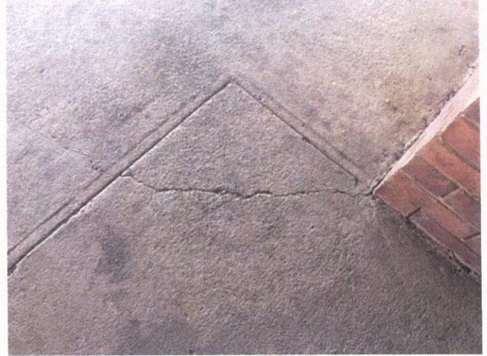
Delap cracks to concrete
