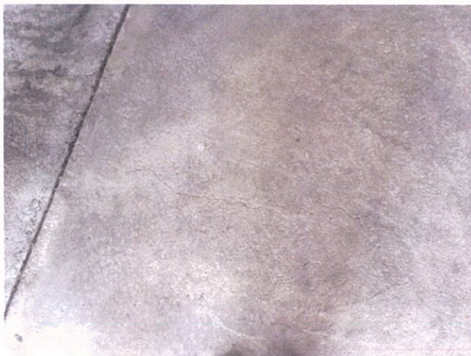
Delap cracks to concrete
