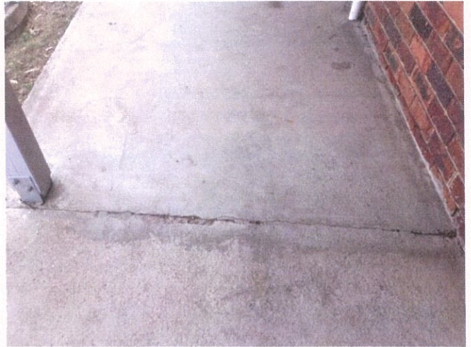
Delap cracks to concrete
