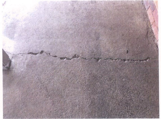
Delap cracks to concrete
