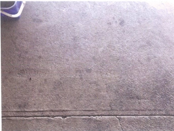
Delap cracks to concrete
