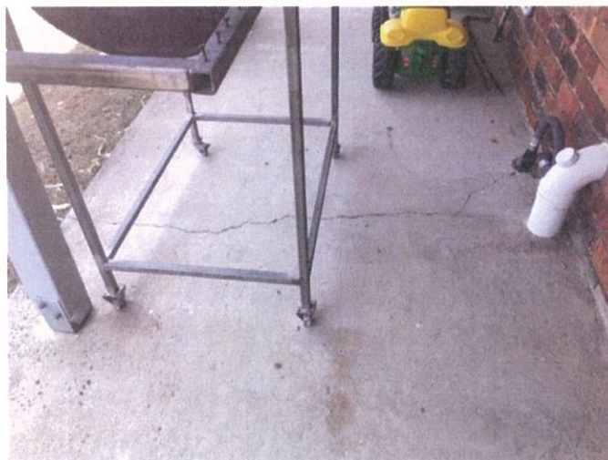
Delap cracks to concrete
