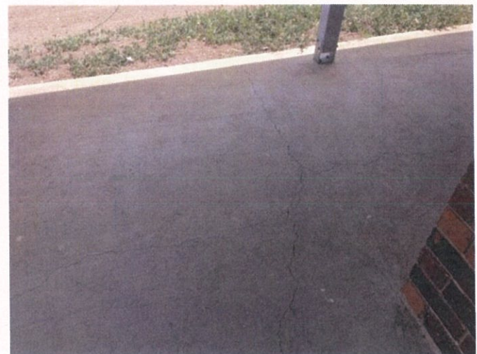
Delap cracks to concrete
