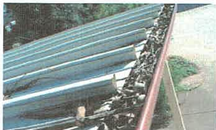
1. A typical suburban gutter clogged with leaf litter prior to cleaning.
