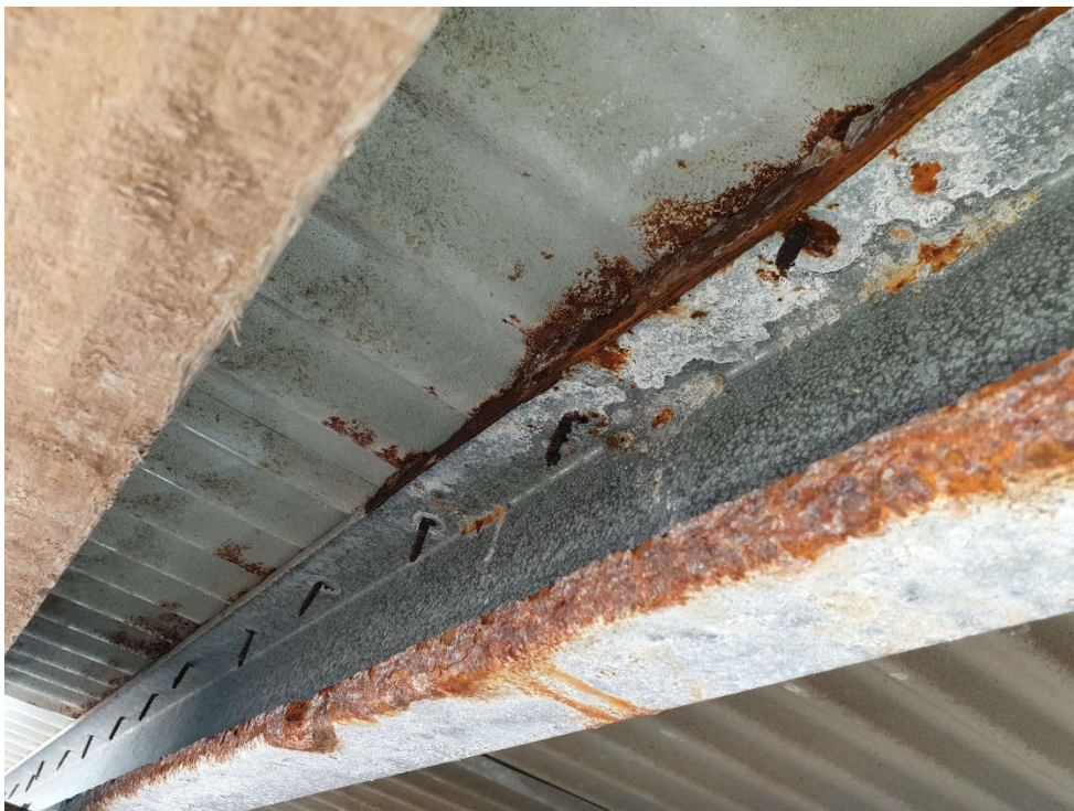
Underside of roof structure severe corrosion requiring replacement.
