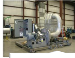
Maintaining exhaust systems on machines
