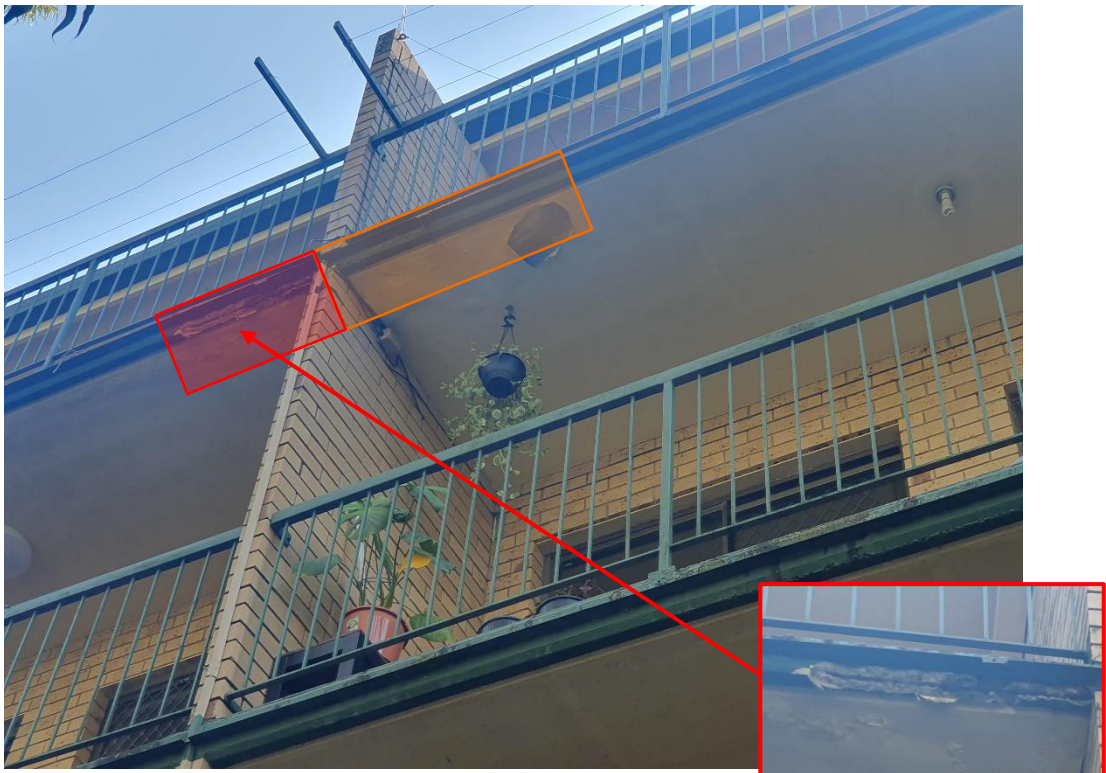
PHOTOGRAPH 40.: Sections/ chunks of concrete slab have fallen away. Large areas of reinforcement reinforcement corroded/ exposed
