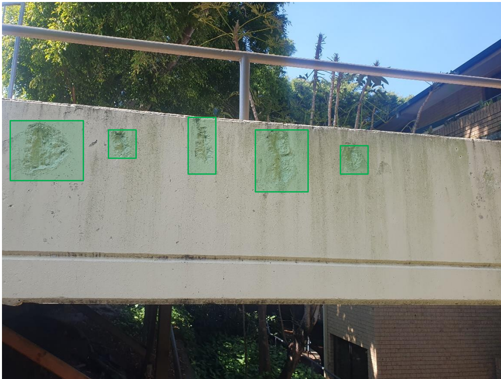
PHOTOGRAPH 25.: Spalling of concrete wall over bridge, evident of concrete blow out due to concrete cancer
