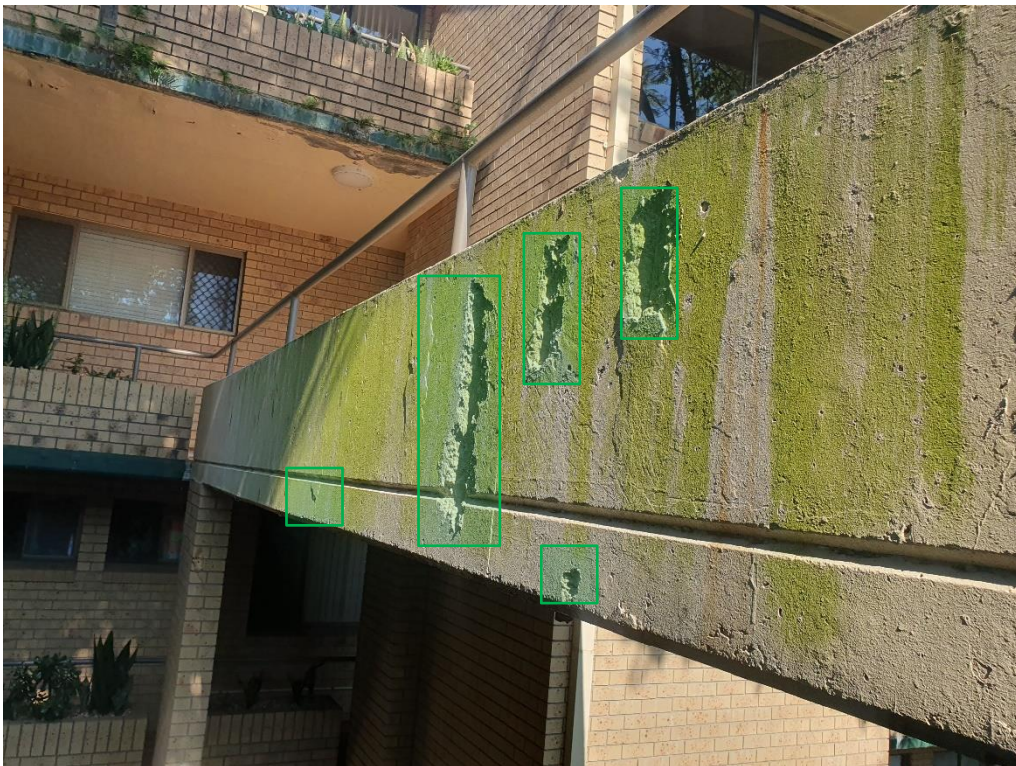
PHOTOGRAPH 22.: Spalling of concrete wall over bridge, evident of concrete blow out due to concrete cancer
