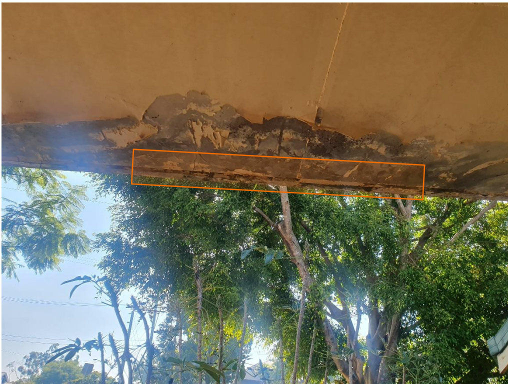
PHOTOGRAPH 12.: cracking to concrete slab, spalling to some areas.
