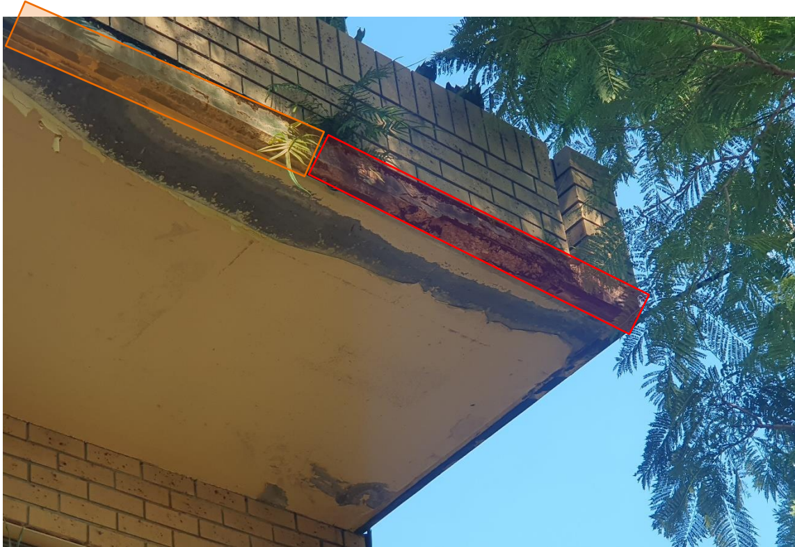
PHOTOGRAPH 5.: Moderate concrete cancer 2.0m from corner along balcony.
