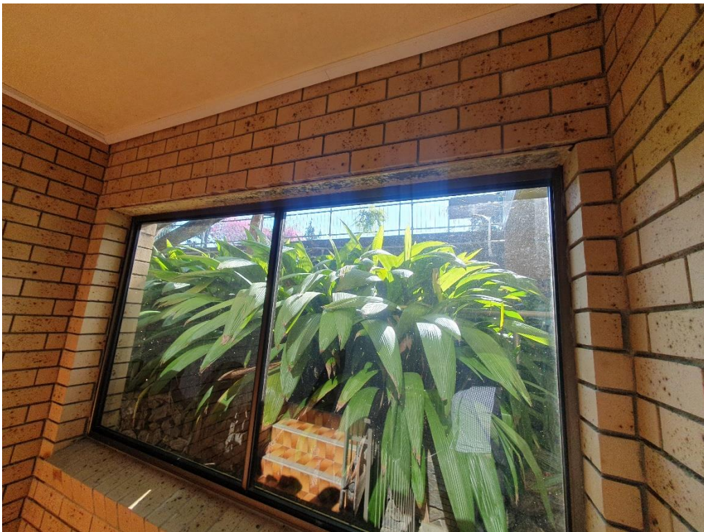
PHOTOGRAPH 20.: Minor corrosion to steel window lintel
