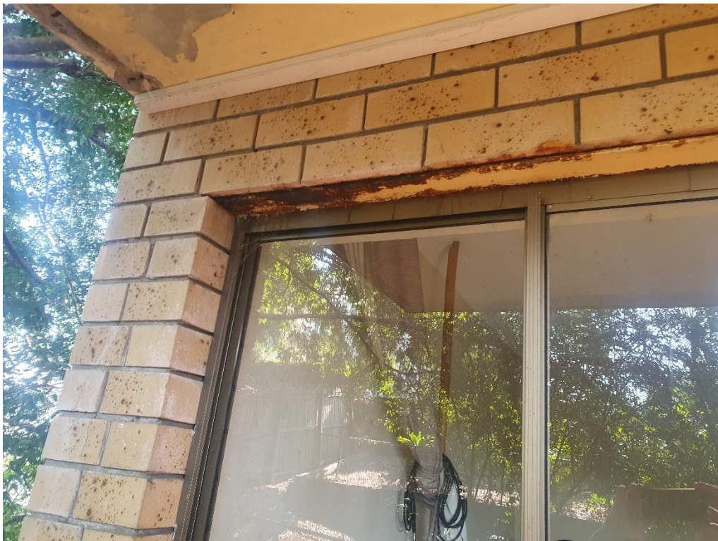
PHOTOGRAPH 16.: Moderate corrosion to steel window lintel
