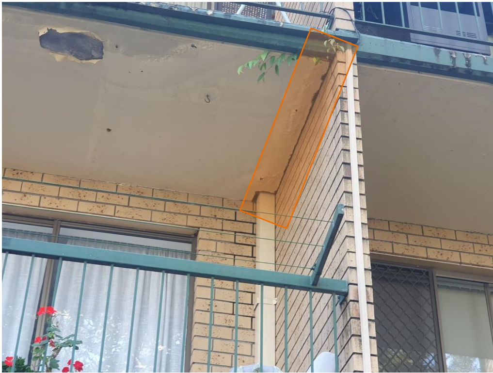
PHOTOGRAPH 35.: Concrete slab expansion alongside brick support
