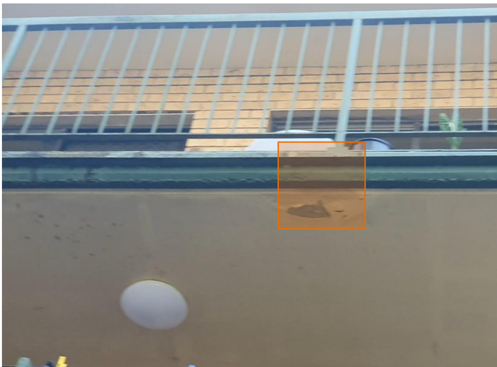
PHOTOGRAPH 32.: Minor spalling/ blow out of concrete slab
