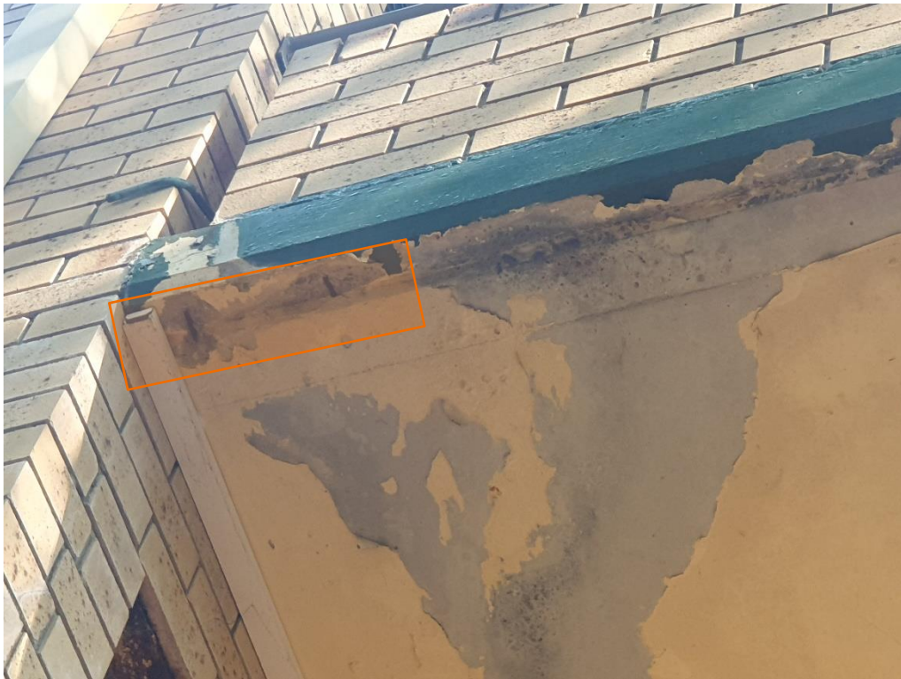
PHOTOGRAPH 15.: Small area of exposed reinforcement, some minor slab spalling/ deterioration
