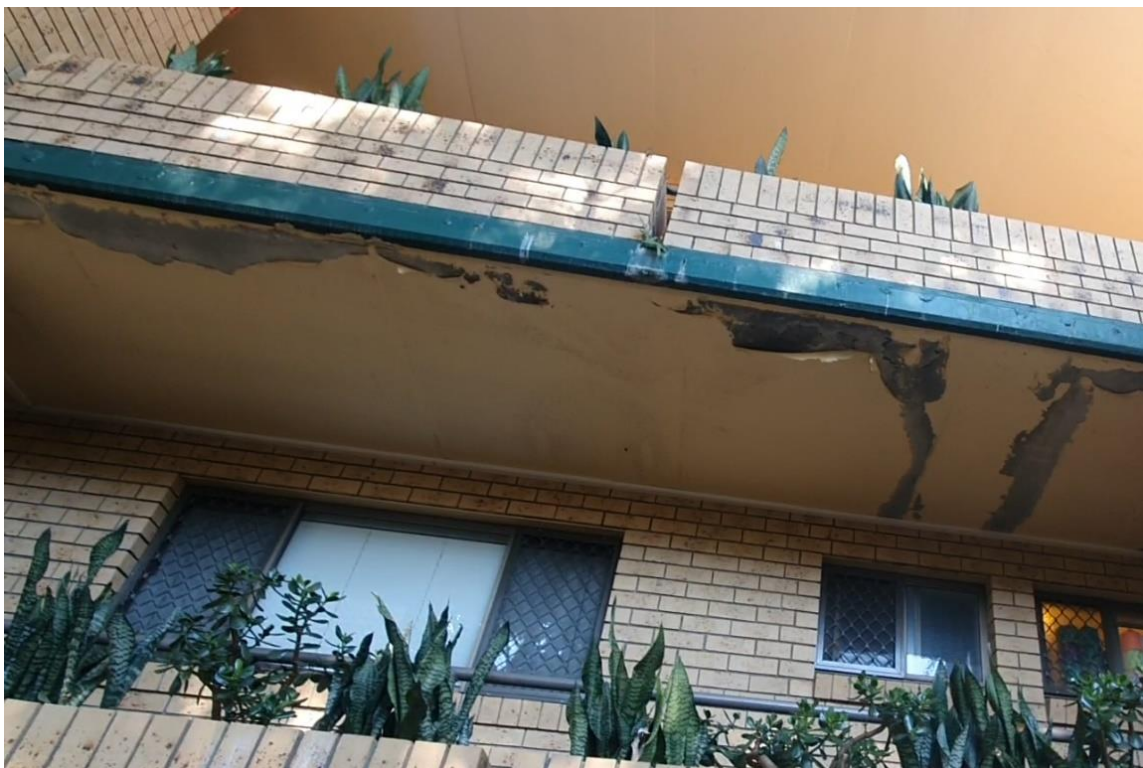
PHOTOGRAPH 8.: LHS – paint peeling/ spalling, concrete generally in good condition RHS – Concrete spalling, some voids to reinforcement
