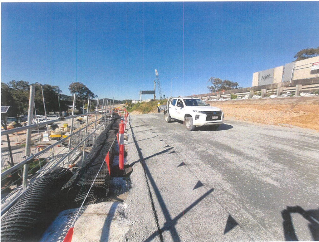
Photo 2. Some minor deformation was observed on one area of the platform.
