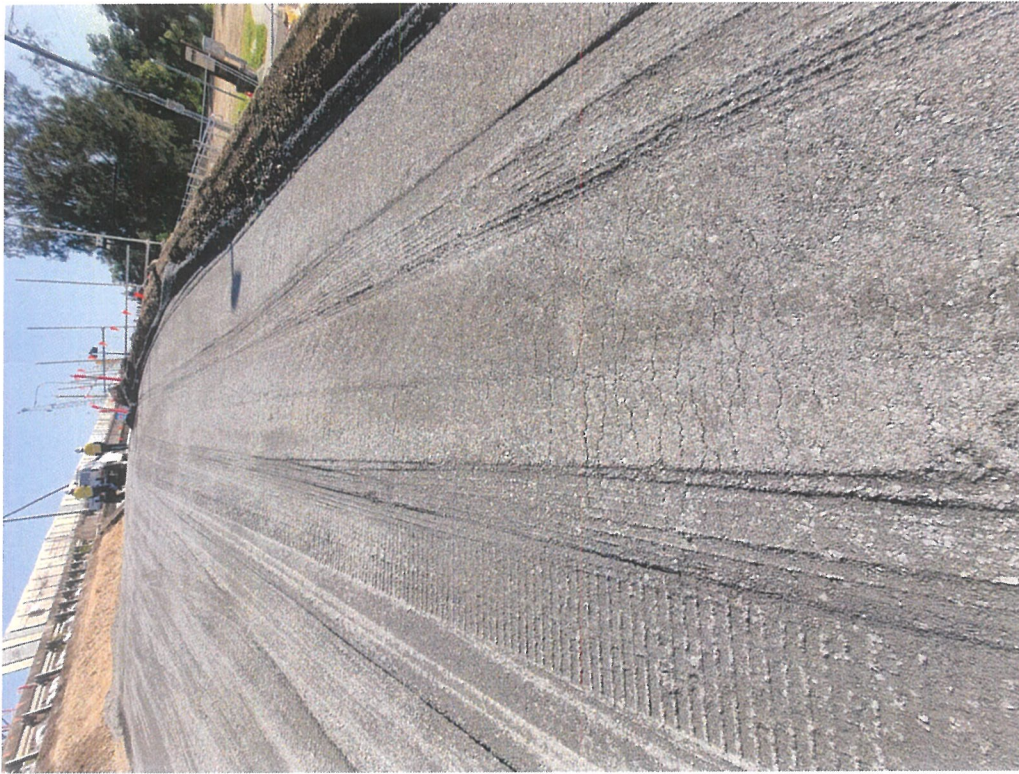
Photo 3. Material on the ramp was observed not to be well compacted. During the proof roll test heaving and deflection was observed along the ramp.
